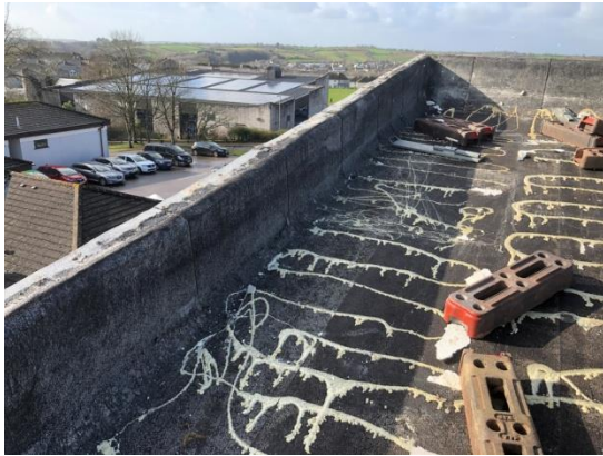
south west bay to roof following strip back of damaged roofing material, insulation and edge trim
