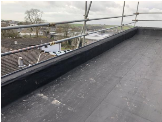
south west bay to roof following strip back of damaged roofing material, insulation and edge trim
