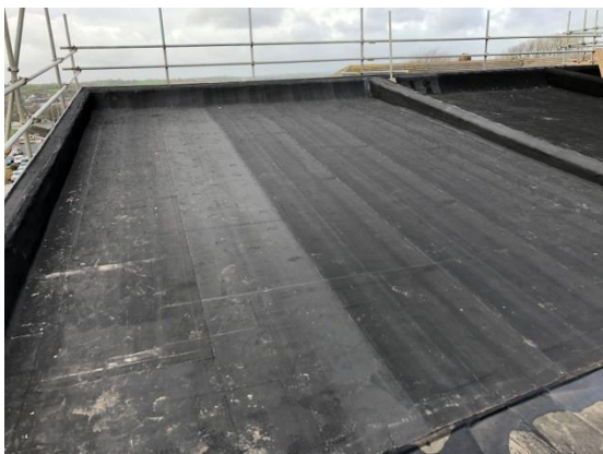
south west bay to roof following strip back of damaged roofing material, insulation and edge trim
